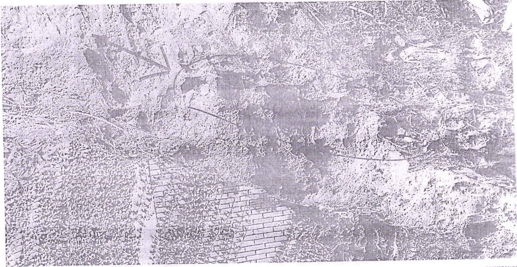
Photo 3: 24 Jan 2020, In addition to the crack, settlement of soil mass is seen in the dumped portion leaving a gap with the upright slope. This might be due to consolidation of soil due to rain.
