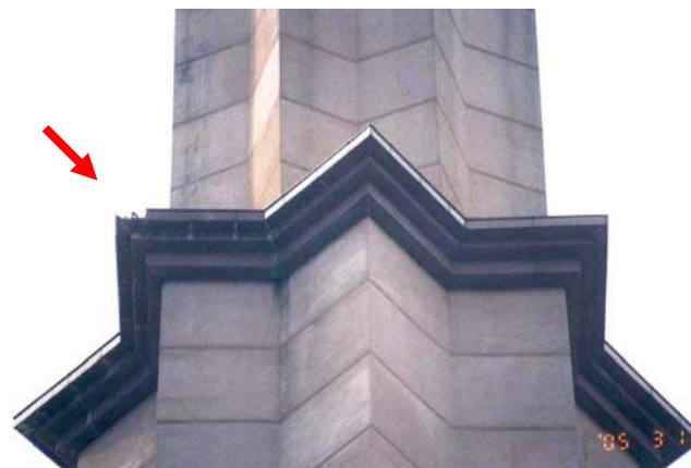
Fig. 7: Close-up view of the lightning damaged section of the minaret (arrowed).
