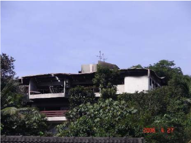
Fig. 3: The fire damaged top floor of a house that was struck by lightning.
