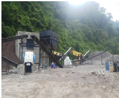
Crusher Plant at Shaktikhor(NCB-09)
