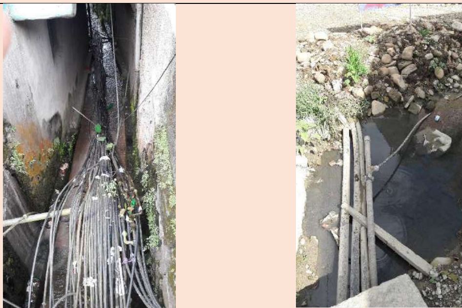
(a) Vulnerable drinking water supply pipelines along drainage in Putalibazar
